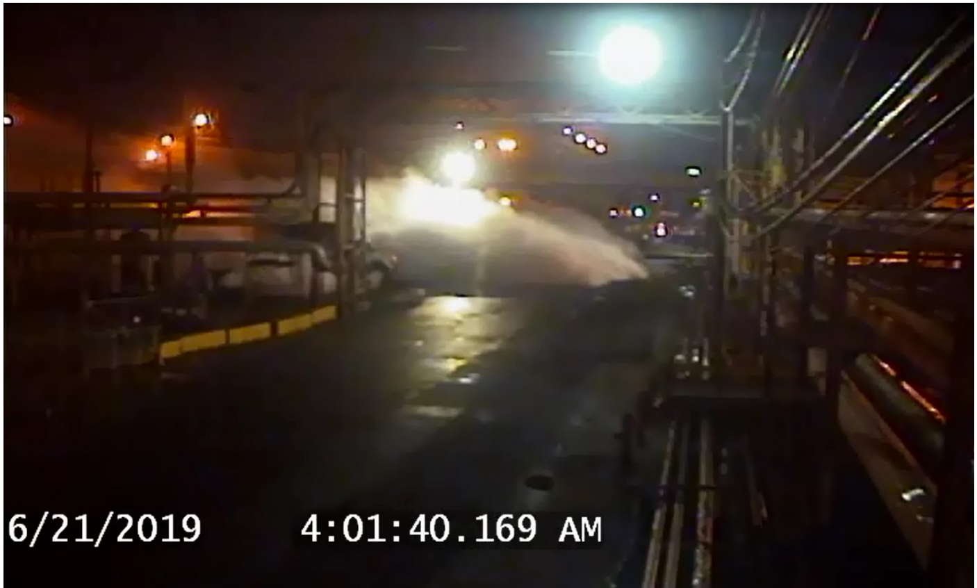
Figure 3. Security camera footage of leaking process fluid. It formed a large ground-hugging vapor cloud that surrounded some sections of the unit. (Credit: PES).
